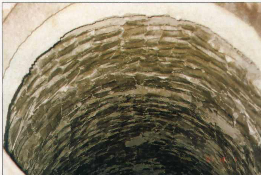
Leaks that have not resulted in structural erosion can be sealed with water plug or chemical grouts.
